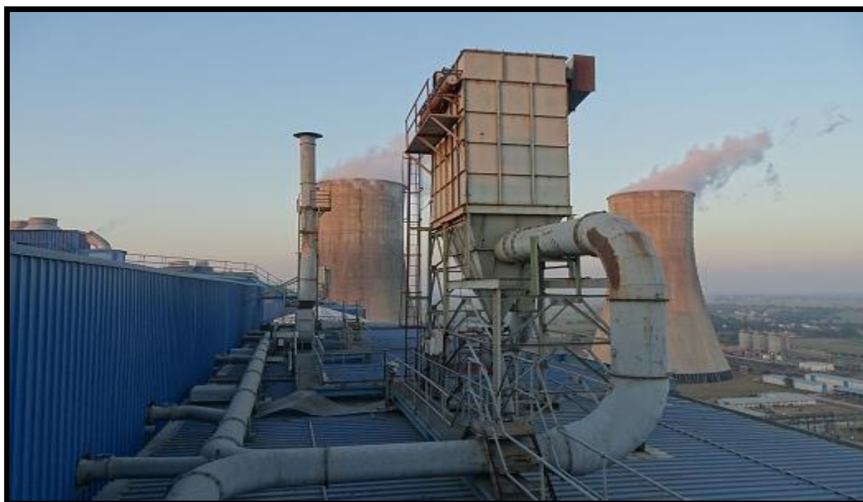
Dust Extraction System at Bunker
