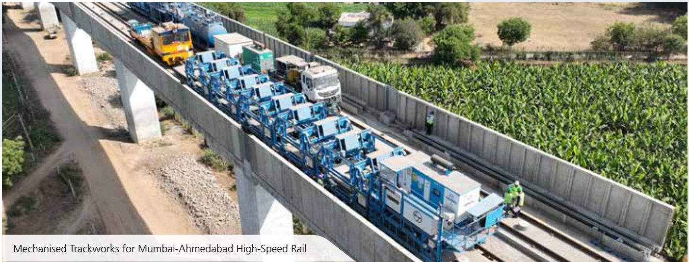
Precast slab track, Delhi-Meerut Regional Rapid Transit System
